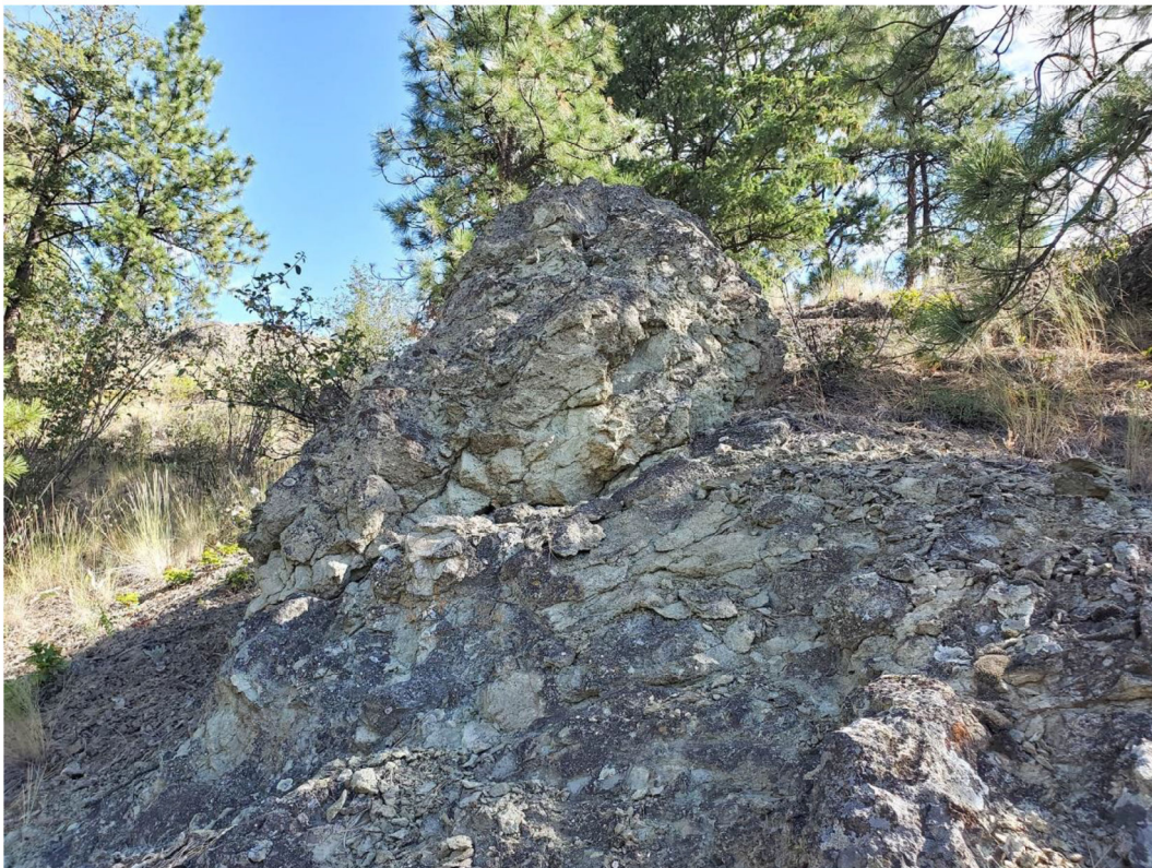
Figure 7B. Loose rock near the eastern side of 1490 Cara Glen Way.
